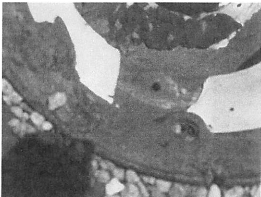
Photo #3: Bolts are not lined up, somehow the drain shifted or was never clamped down to begin with.
