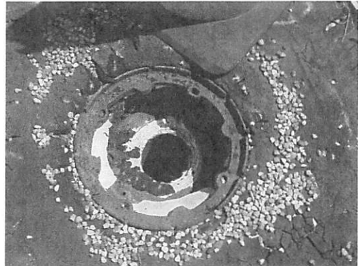
Photo #2: Drain is not clamped down on the West side of Section E
