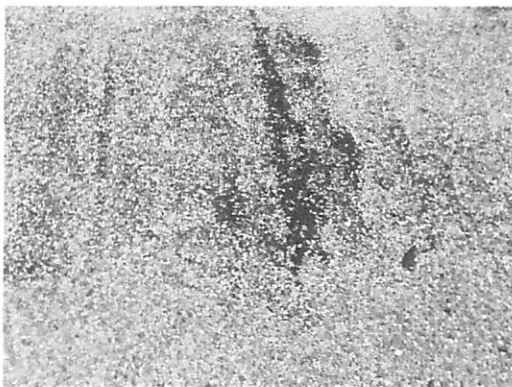
Photo #5: Eroded felts throughout all sections
