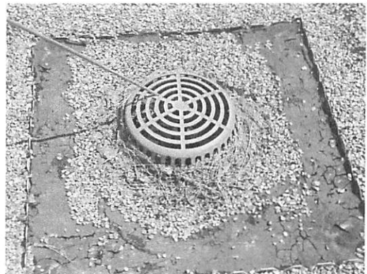
Photo #4: Debris along the drain, again on Section E and throughout
