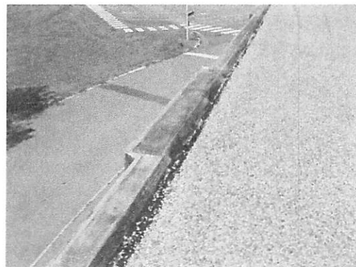
Photo #6: Faded aluminum coating along the East side perimeter on Section B
